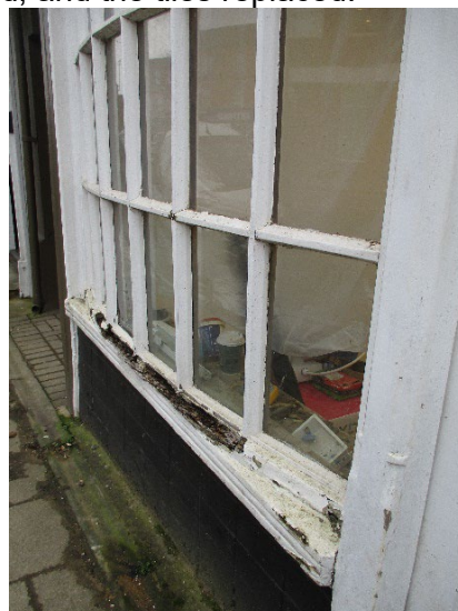
The woodwork is not in good condition
