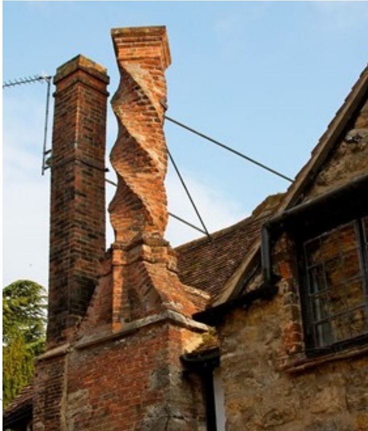
Historic twisted chimney attached to grade 2* listed building and dating from the 16th century.
